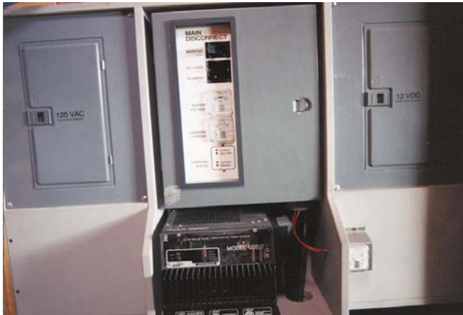
Above: Inverter, instrumentation, and breakers.
